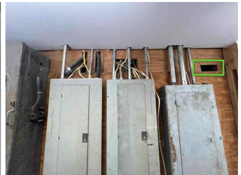
Rear Cross Hallway, Swab Sample Taken Through Openings in Wall
