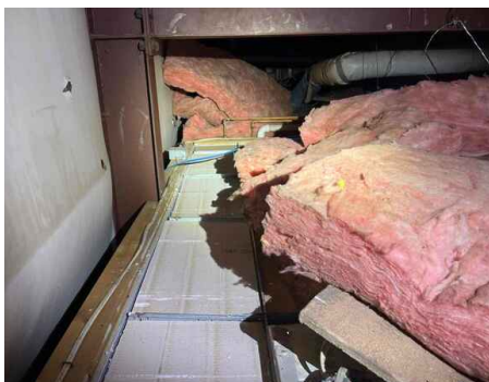
Insulation Above Ceiling Tiles Improperly Installed - Example
