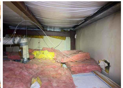
Insulation Above Ceiling Tiles Improperly Installed - Example
