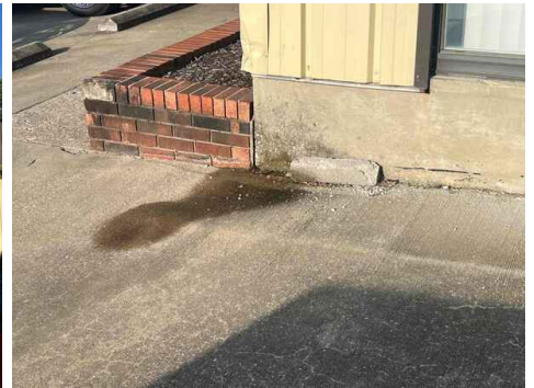
Right Side of Office, Gutters and Facade Leaking - Example
