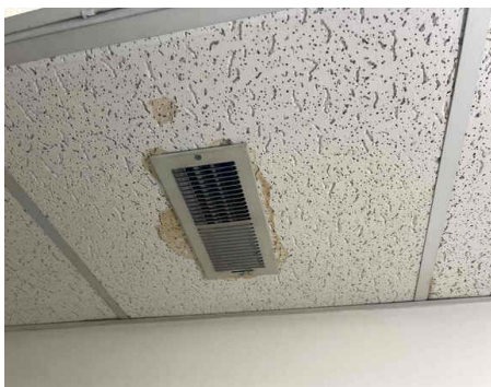
Break Room, Ceiling Stains - Dry
