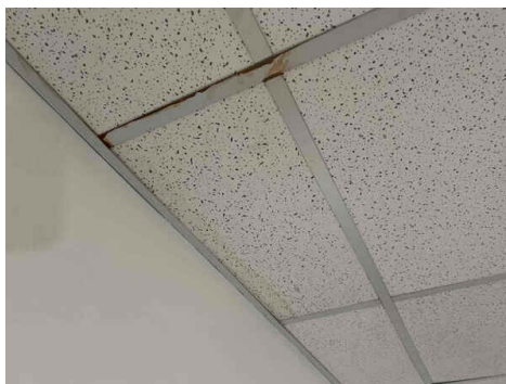
Hallway, Ceiling Stains - Dry
