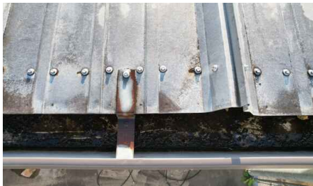
Left Gutters, Appear to Have Been Cleaned of Large Debris Only
