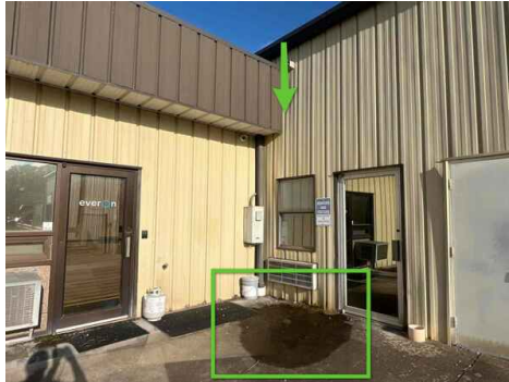
Right Side of Office, Warehouse Gutters Leaking
