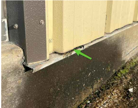
Right Side of Office, Water Behind Siding (From Gutters and Facade Leaking
