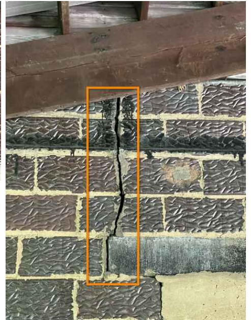
Wall Crack - Example
