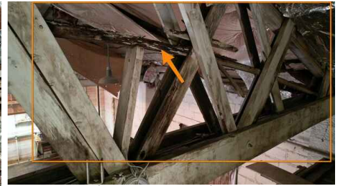
Main Warehouse, Rotted Truss
