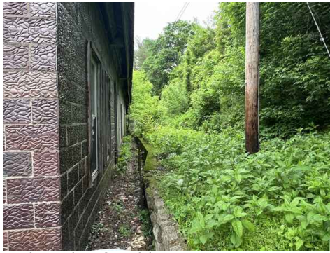
Right Side of Building, Negative Grading, Wet
