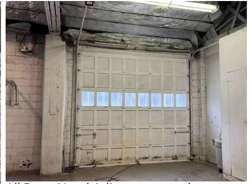
All Door Need Adjustment and Lubrication - Example
