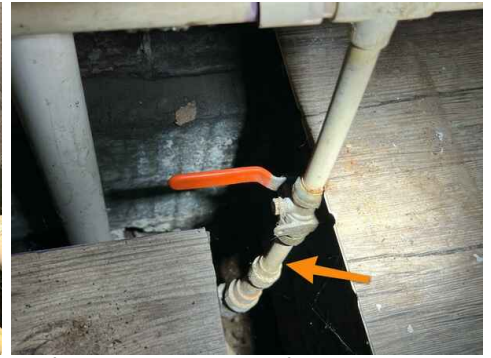
Bathroom, Water Supply Lines, Improperly Installed/ Supported
