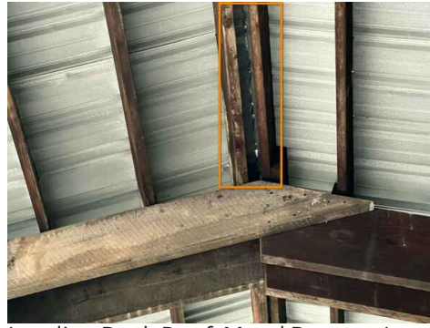
Loading Dock Roof, Metal Damage/ Roof Leaks
