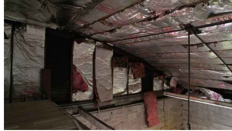
Example of Insulation Failure
