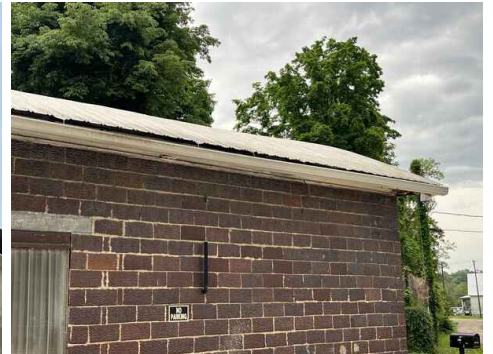
Left Side of Warehouse, Gutter and Downspout Damaged
