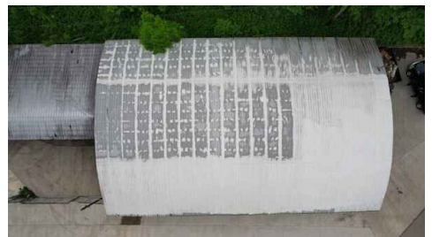
Trees Overhanging Roof, Potential for Damage and Gutters Being Clogged
