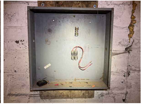
Rear Warehouse Space Electrical Panels
