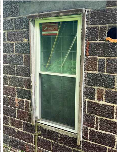
Example of Exterior Wood Component Deterioration
