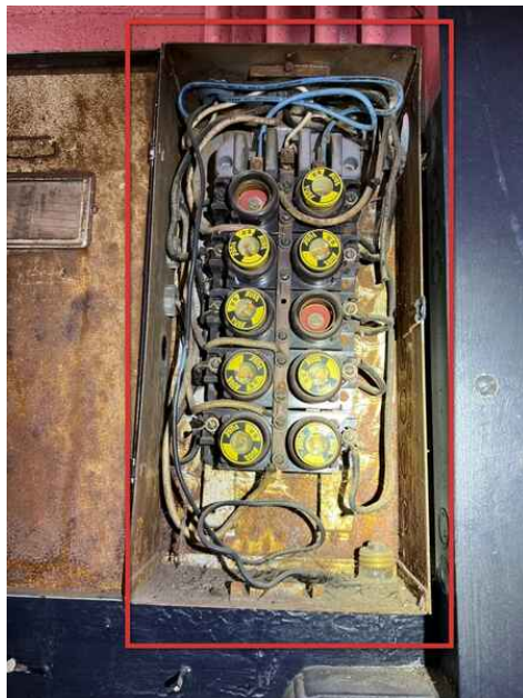
Fuse Panel, Recommend Replacement
