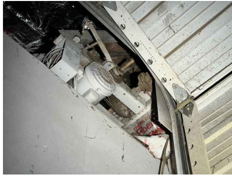
Rear Garage Door Opener, Not Connected, Operated When Tested
