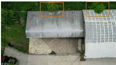
Trees Overhanging Roof, Potential for Damage and Gutters Being Clogged
