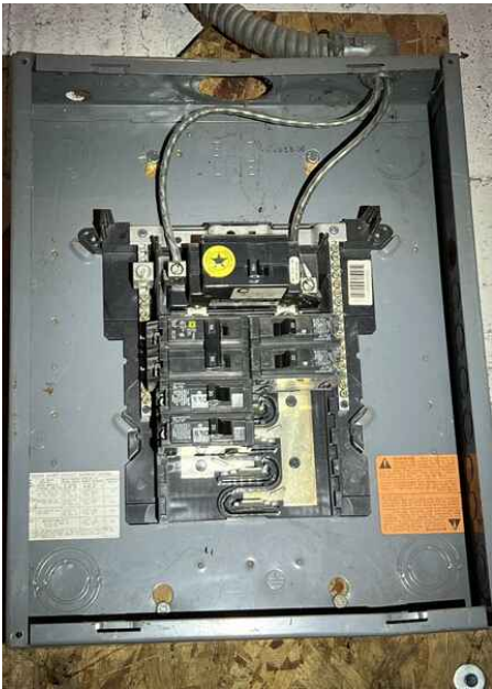
Rear Warehouse Space Electrical Panels
