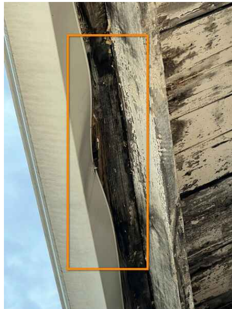
Left Side of Warehouse, Gutter and Downspout Damaged
