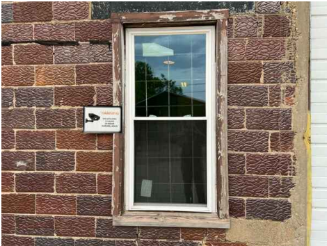
Example of Exterior Wood Component Deterioration
