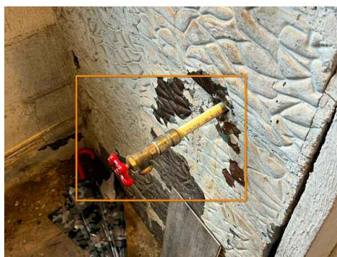
Bathroom, Water Supply Lines, Improperly Installed/ Supported
