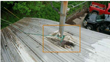
Warehouse Roof, Flashing Deterioration
