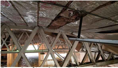
Example of Insulation Failure
