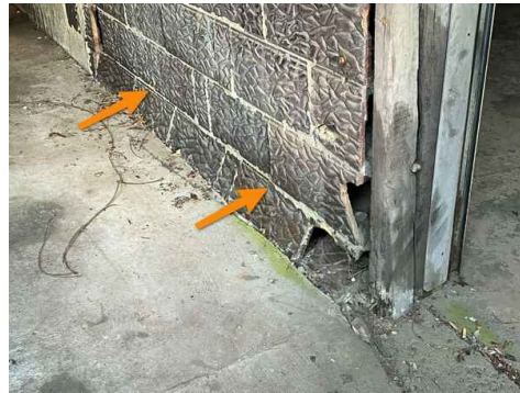
Wall Crack - Example
