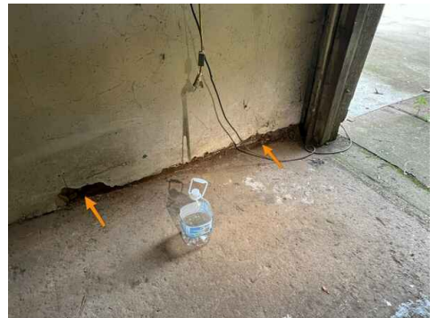
Wall Damage, Rear Warehouse Space, Water Intrusion
