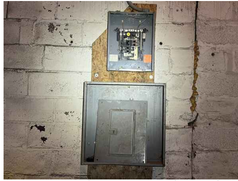
Rear Warehouse Space Electrical Panels
