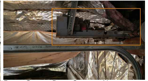
Front Garage Door Opener, Not Connected to Door, Not Tested
