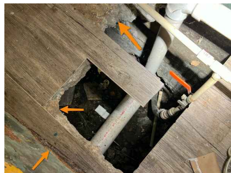
Bathroom, Example of Floor Rot/ Deterioration
