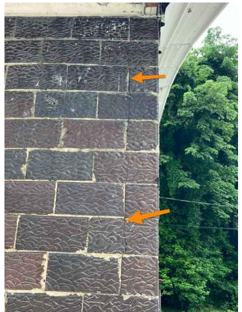
Wall Crack - Example
