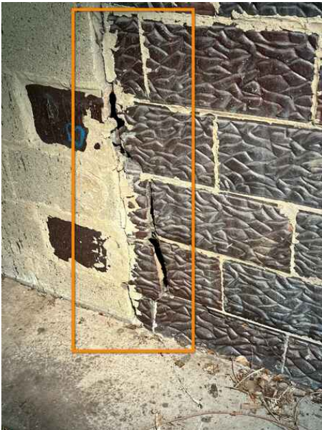
Wall Crack - Example
