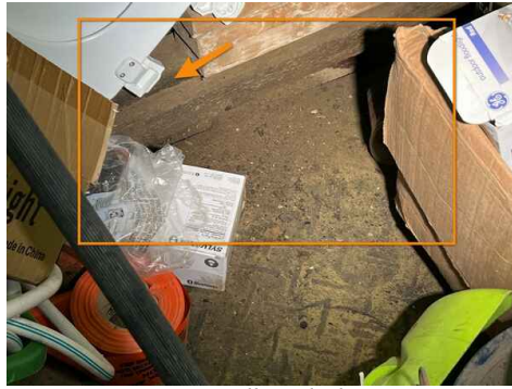
Storage Room, Wall and Floor Wet, Dirt Coming in From Outside
