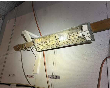
Rear Warehouse Space Lighting Example
