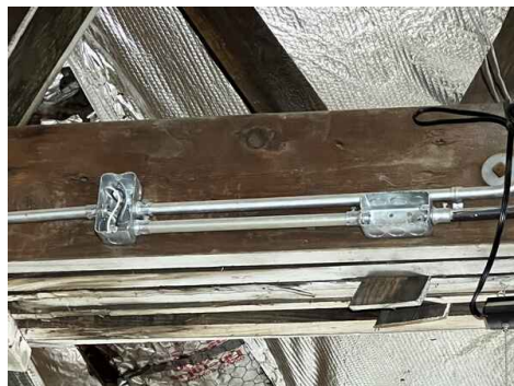
Additional Junction Boxes Missing Covers
