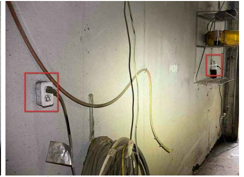
Example of Receptacles Not GFCI Protected (20-30+)
