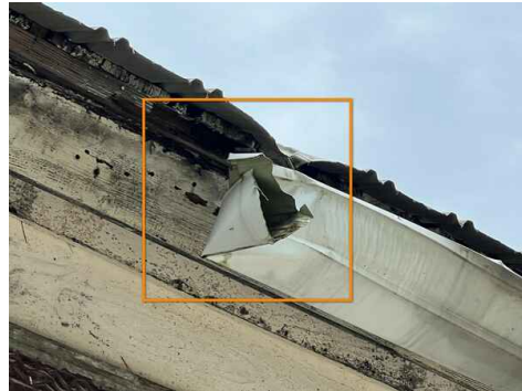
Left Side of Warehouse, Gutter and Downspout Damaged
