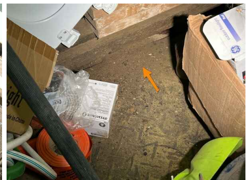
Storage Room, Evidence of Active Water Intrusion - Wet
