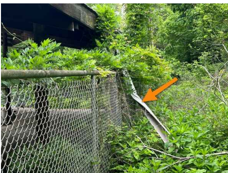
Right Side of Loading Dock Area, Gutter and Downspout Damaged
