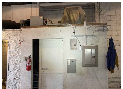
Main Warehouse Panel
