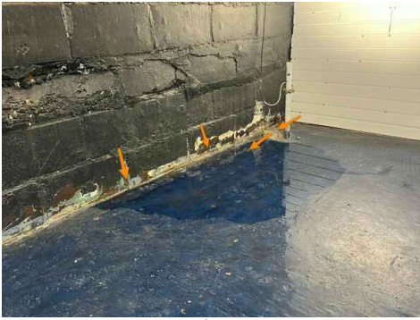
Party Room - Standing Water
