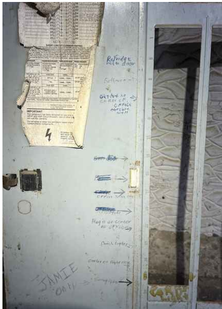
Main Warehouse Panel
