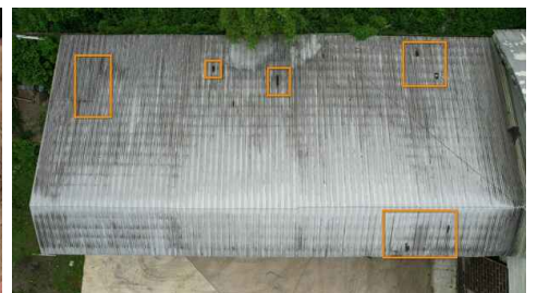
Loading Dock Roof, Metal Damage/ Roof Leaks
