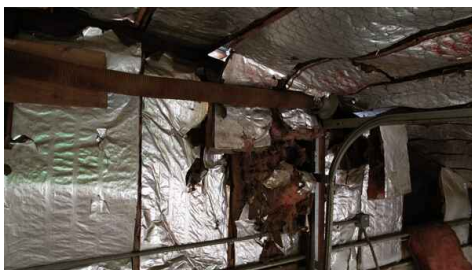
Example of Insulation Failure
