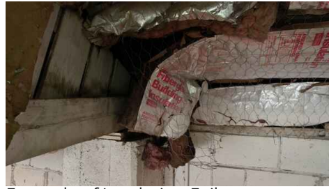
Example of Insulation Failure
