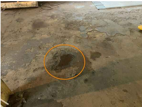
Example of Active Roof Leak Water Intrusion
