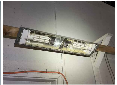
Rear Warehouse Space Lighting Example
