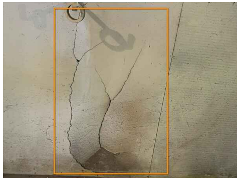
Example of Cosmetic Wall Damage
