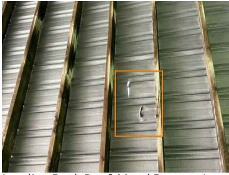
Loading Dock Roof, Metal Damage/ Roof Leaks
