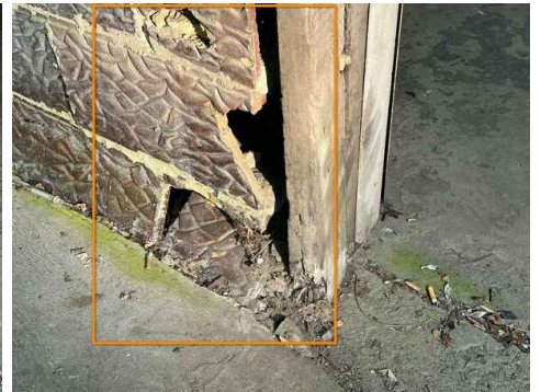
Wall Crack - Example
