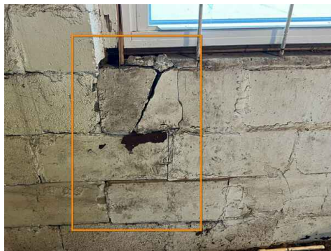
Wall Crack - Example
