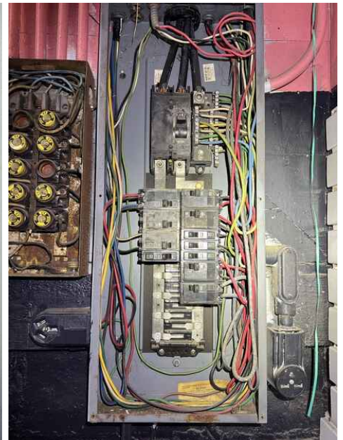
"Party Room" Electrical Panels
