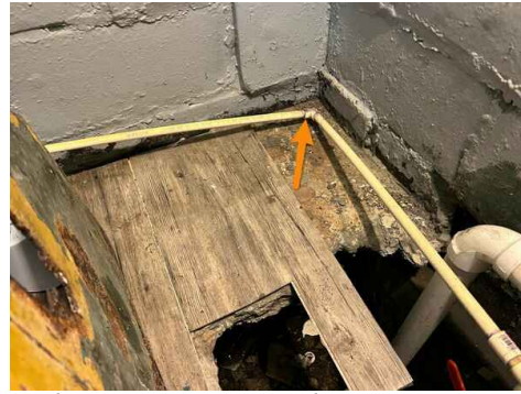
Bathroom, Water Supply Lines, Improperly Installed/ Supported
