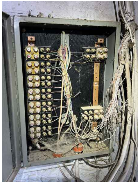
Main Warehouse Telephone Junction Panel
