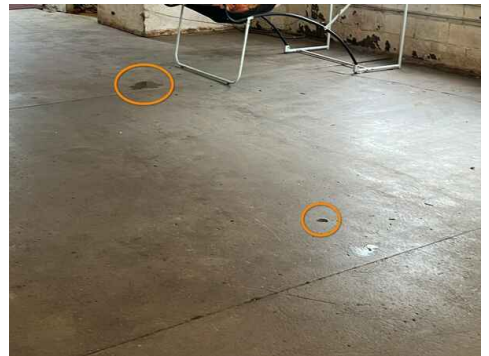
Example of Active Roof Leak Water Intrusion
