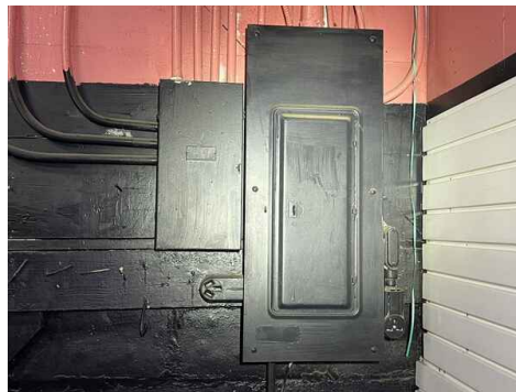
"Party Room" Electrical Panels
