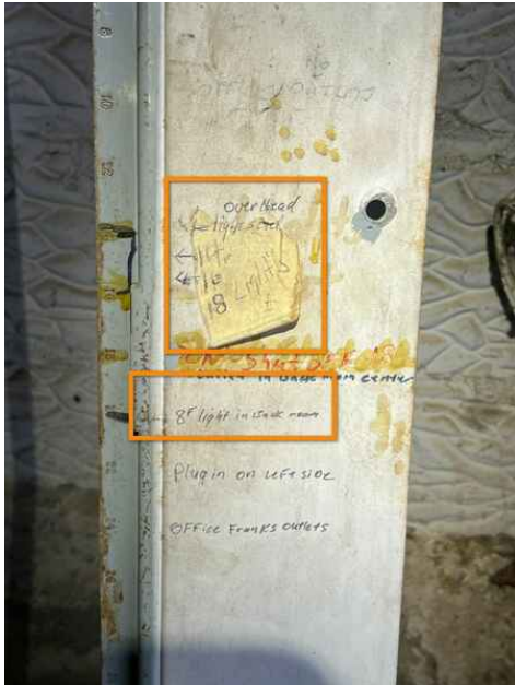
Front Door Panel, Most Lights Controlled by Breakers
