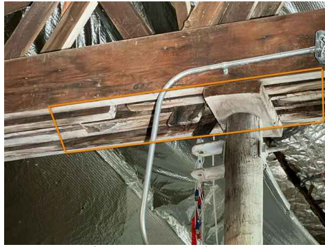
Main Warehouse, Rotted Truss, Supported By Post
