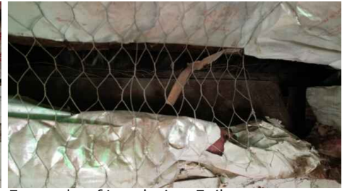
Example of Insulation Failure
