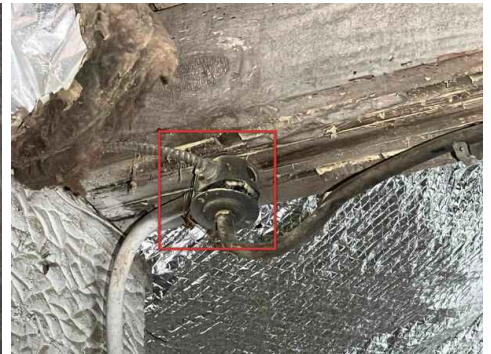
Electrical Junction Box Open, Potential for Water or Pest Intrusion
