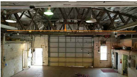
Main Warehouse, Rotted Truss
