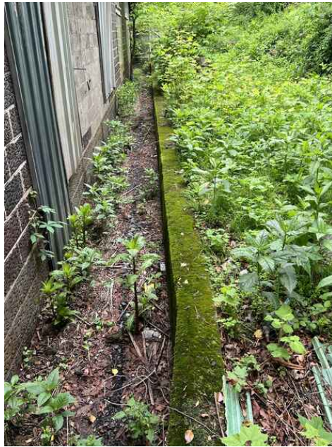
Right Side of Building, Negative Grading, Wet
