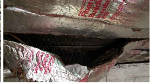
Example of Insulation Failure
