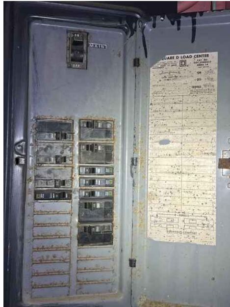
"Party Room" Electrical Panels
