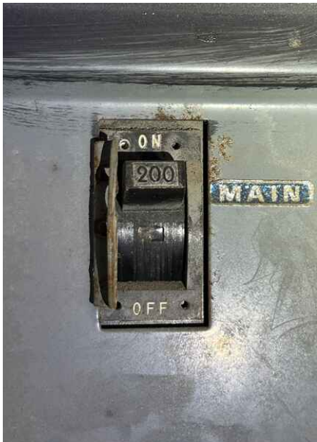
"Party Room" Electrical Panels
