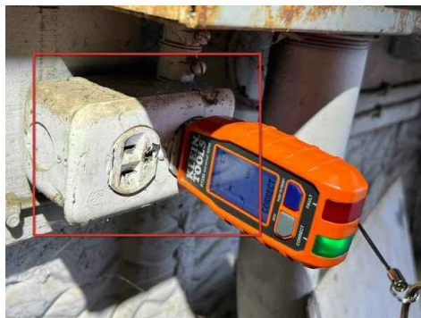
Example of Receptacles Not GFCI Protected (20-30+)
