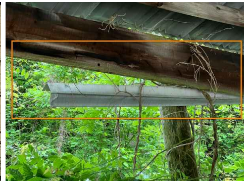
Right Side of Loading Dock Area, Gutter and Downspout Damaged
