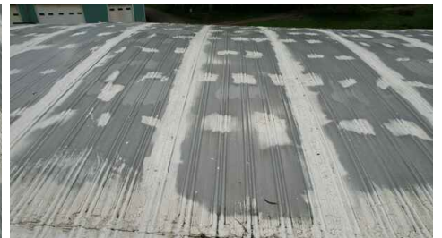
Warehouse Roof, Metals Seams and Fasteners Need Sealed
