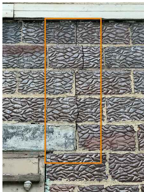
Wall Crack - Example
