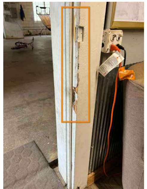
Office Door, Frame Damaged
