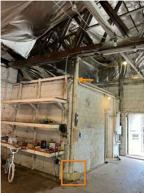
Main Warehouse, Rotted Truss, Supported By Post
