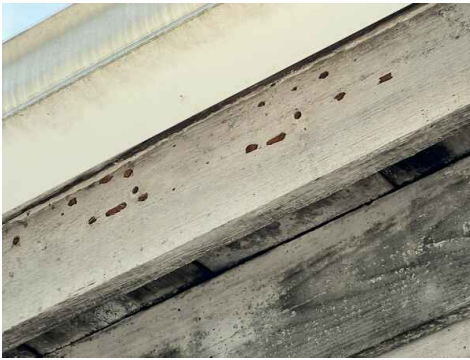
Left Side of Warehouse, Carpenter Bee Damage - Example
