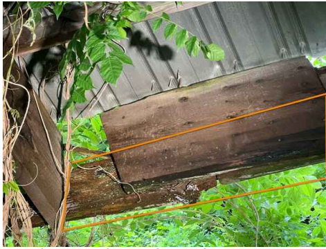
Loading Dock Roof, Roof Framing, Rotted Wood
