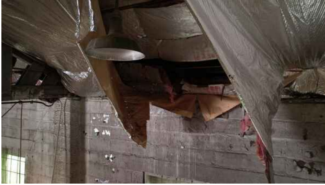
Example of Insulation Failure
