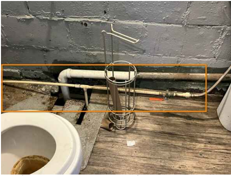
Bathroom, Water Supply Lines, Improperly Installed/ Supported
