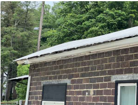
Left Side of Warehouse, Gutter and Downspout Damaged
