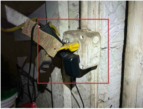
Example of Receptacles Not GFCI Protected (20-30+)
