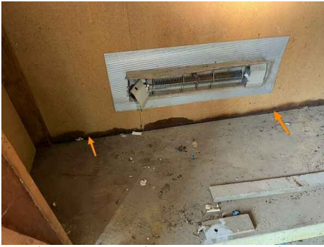
Inside Main Warehouse Storage Closet, Wall Wet, Likely Due to Active Roof Leak
