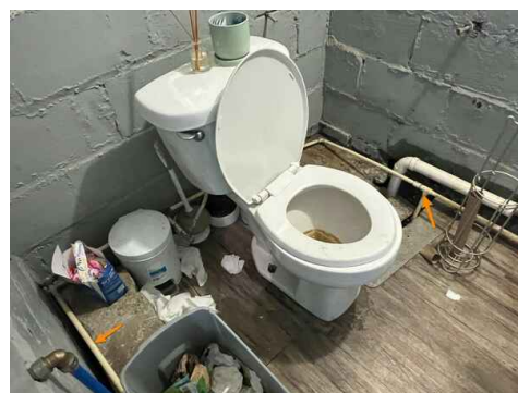
Bathroom, Water Supply Lines, Improperly Installed/ Supported
