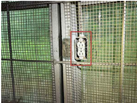
Receptacle Missing Cover - Example
