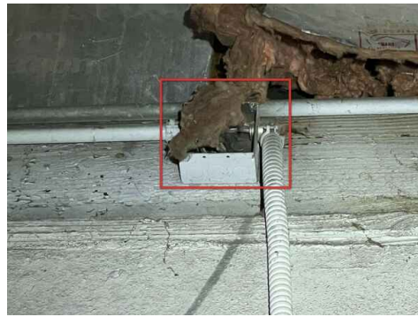
Electrical Box Missing Cover - Example
