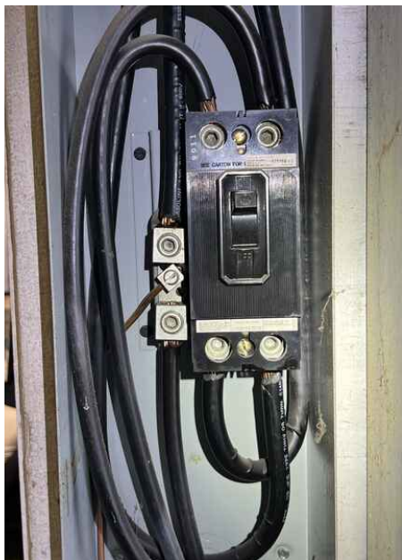
Main Warehouse Panel
