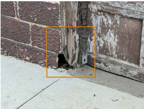
Example of Exterior Wood Component Deterioration
