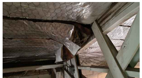
Example of Insulation Failure
