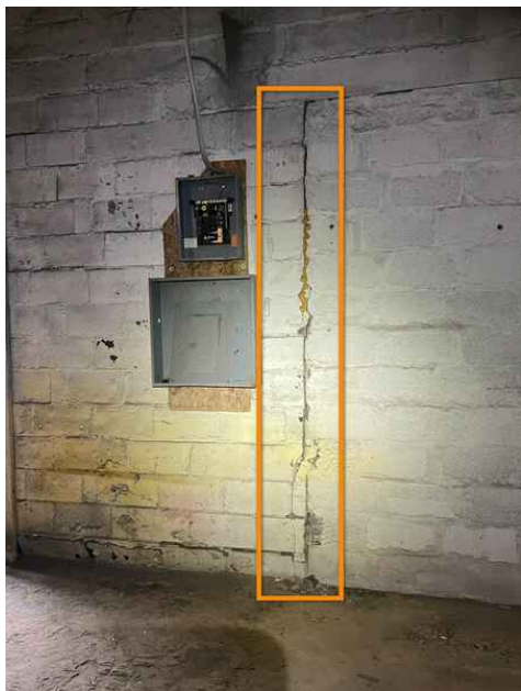
Wall Crack - Example
