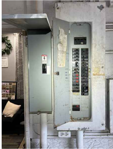
Main Warehouse Panel
