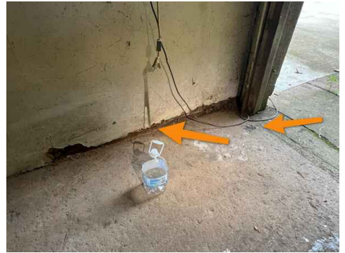
Example of Active Roof Leak Water Intrusion
