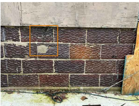
Wall Crack - Example
