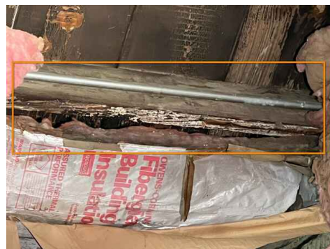
Main Warehouse Roof, Interior Example of Rood Framing Wood Rot
