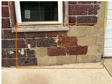
Wall Crack - Example
