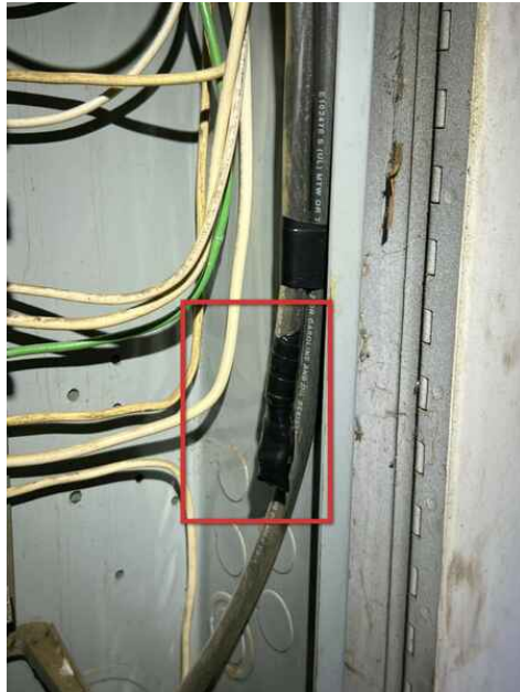
Stray Electrical Panel Wires - Example
