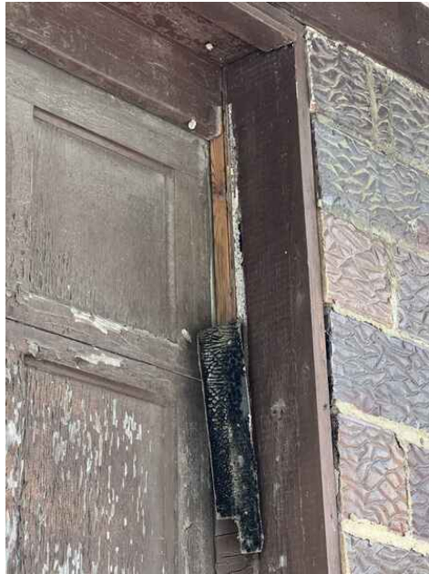
Left Garage Door Deteriorated
