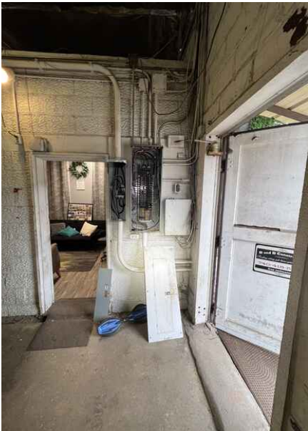
Main Warehouse Panel
