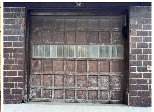
Left Garage Door Deteriorated
