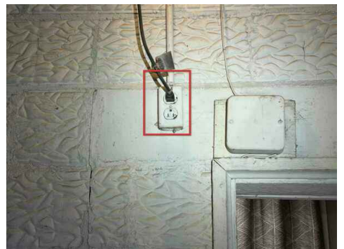
Example of Receptacles Not GFCI Protected (20-30+)
