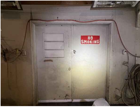
Door to "Party Room", Does Not Operating or Secure Correctly
