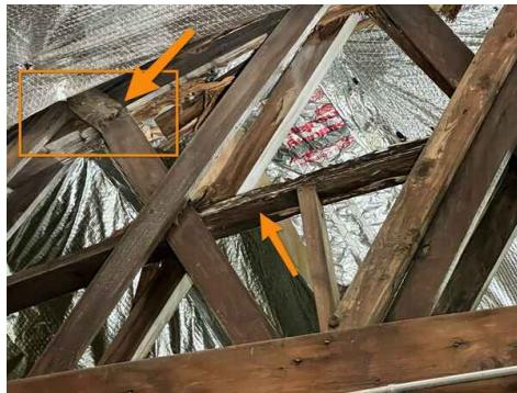
Main Warehouse, Rotted Truss
