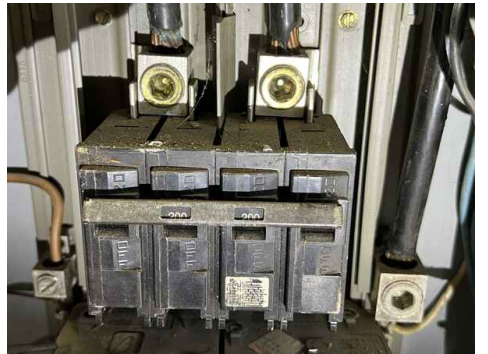
Main Warehouse Panel
