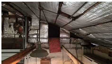
Example of Insulation Failure
