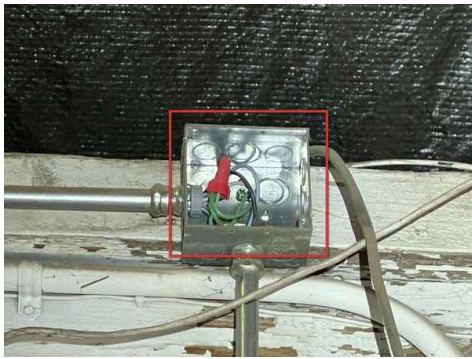
Electrical Box Missing Cover - Example
