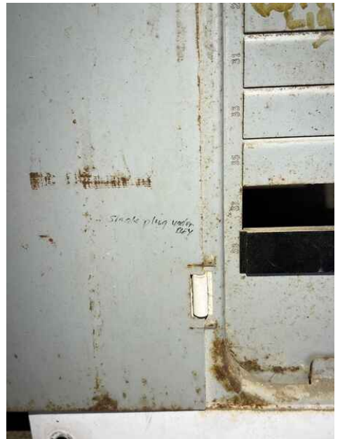
Main Warehouse Panel
