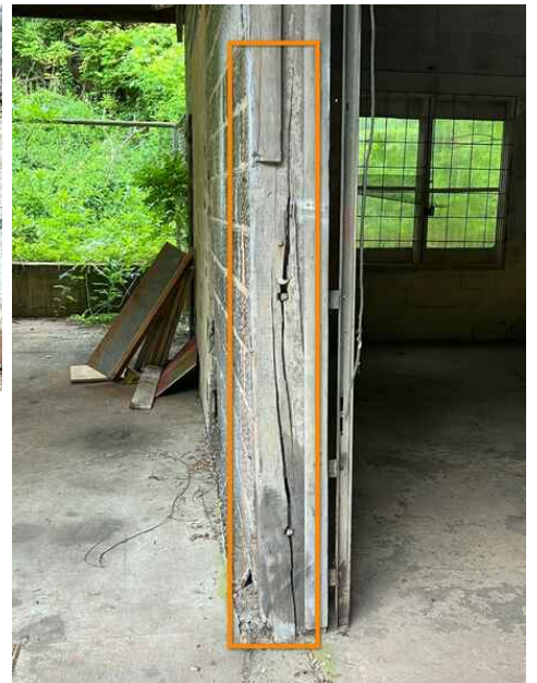
Example of Exterior Wood Component Deterioration
