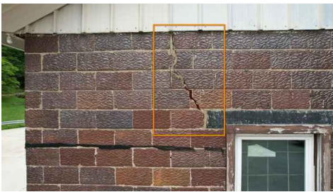
Wall Crack - Example
