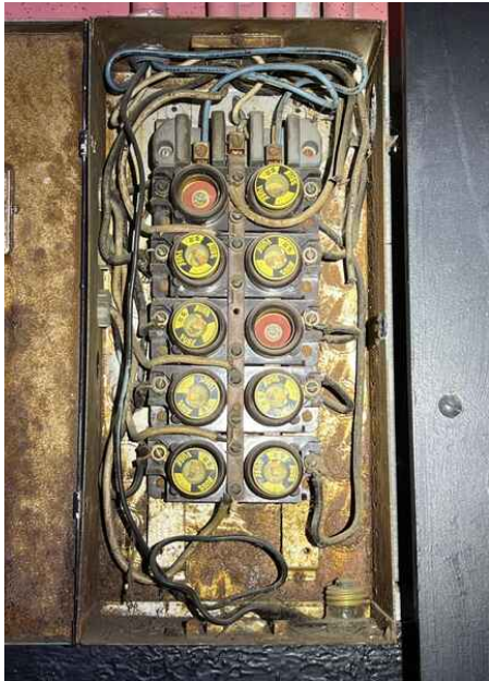
"Party Room" Electrical Panels
