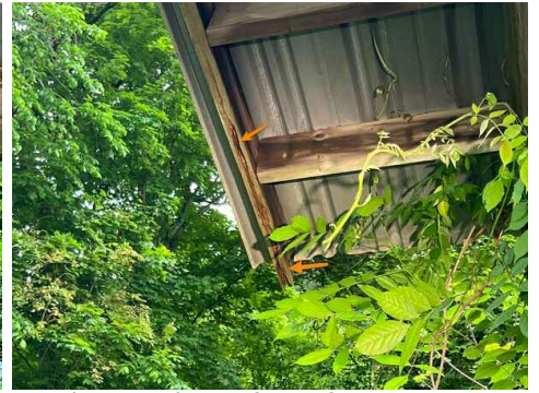
Loading Dock Roof, Roof Framing, Rotted Wood
