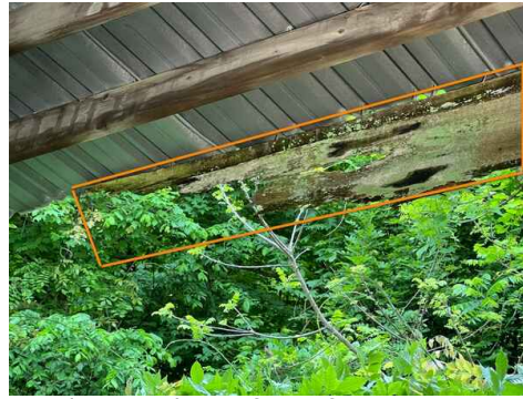
Loading Dock Roof, Roof Framing, Rotted Wood
