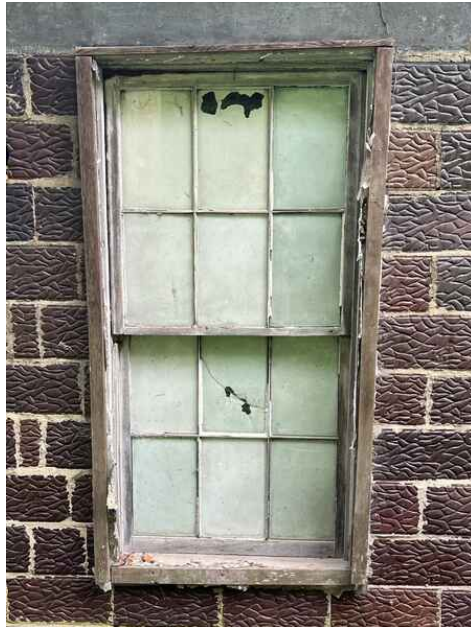
Example of Exterior Wood Component Deterioration
