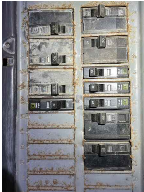
"Party Room" Electrical Panels
