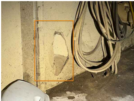
Example of Cosmetic Wall Damage
