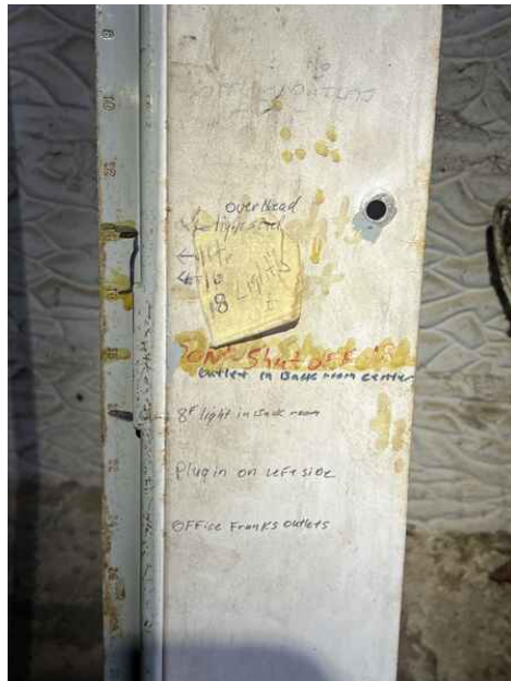
Main Warehouse Panel
