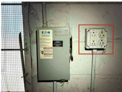
GFCI Fails When Tested
