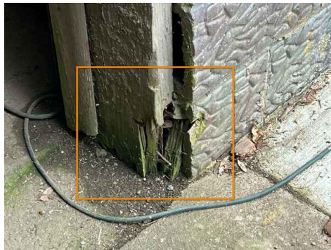
Example of Exterior Wood Component Deterioration
