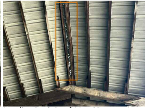
Loading Dock Roof, Metal Damage/ Roof Leaks
